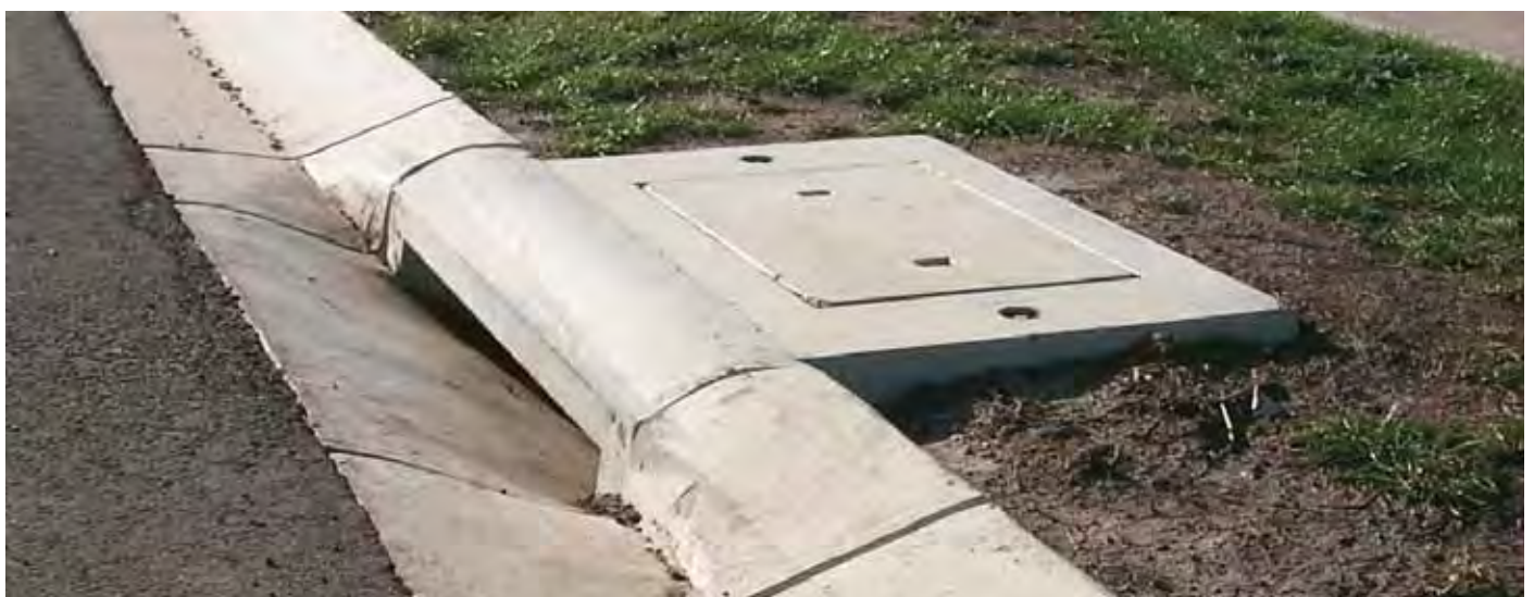
A side entry concrete frame and insert and a concrete kerb lintel installed over a side entry pit.
