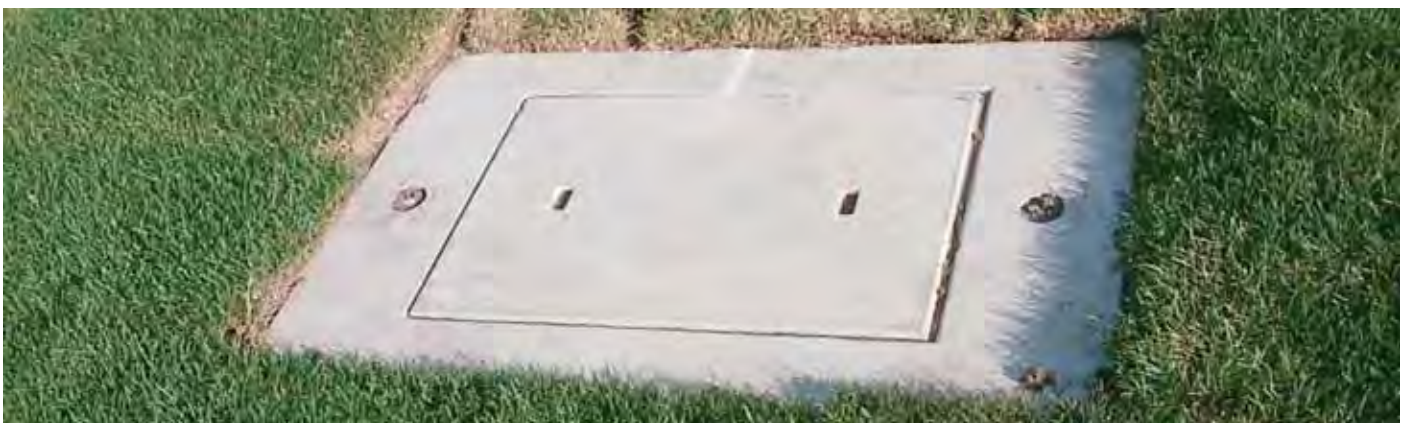
Typical installation of a junction pit concrete frame and insert placed over a junction pit in a nature strip.
